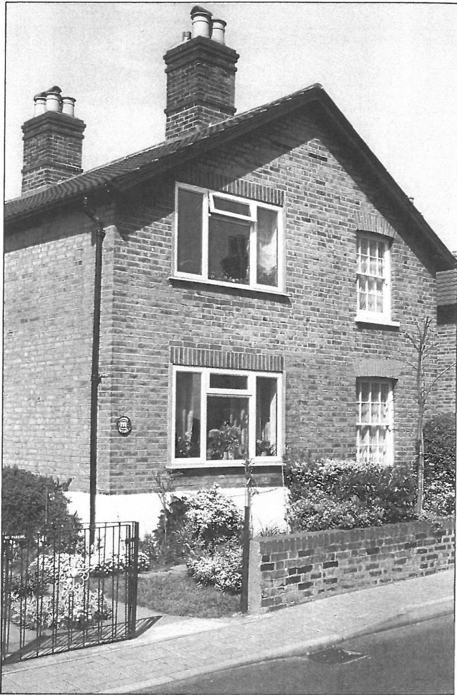
Contrasts in Character A pair of mid Victorian semi-detached houses in the Alexandra Cottage Estate conservation area, Bromley, London. On the left hand side — drastic alterations to the proportions and design of the window openings. On the right, the original recessed timber box sash vertical sliding windows with six over six window panes and glazing bars under curved red gauged brick arched openings.
